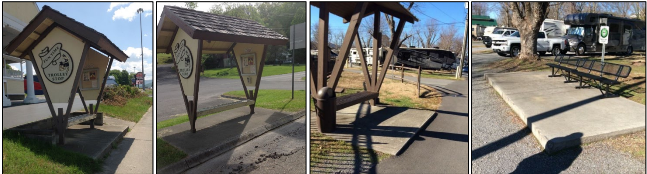
Examples of shelters with vertical displacements at the shelter pad.
