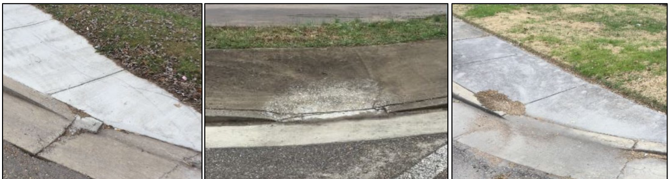
Examples of curb ramps that are less than the minimum 48" width required.
