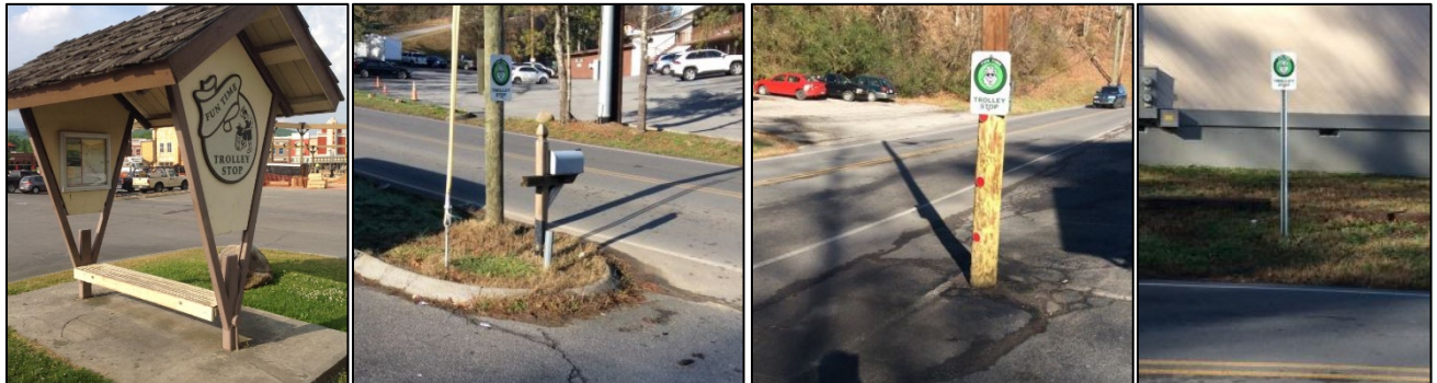
Examples of trolley stops/shelters not located on an accessible route (may also lack a compliant 5' wide x 8' deep boarding/alighting area).
