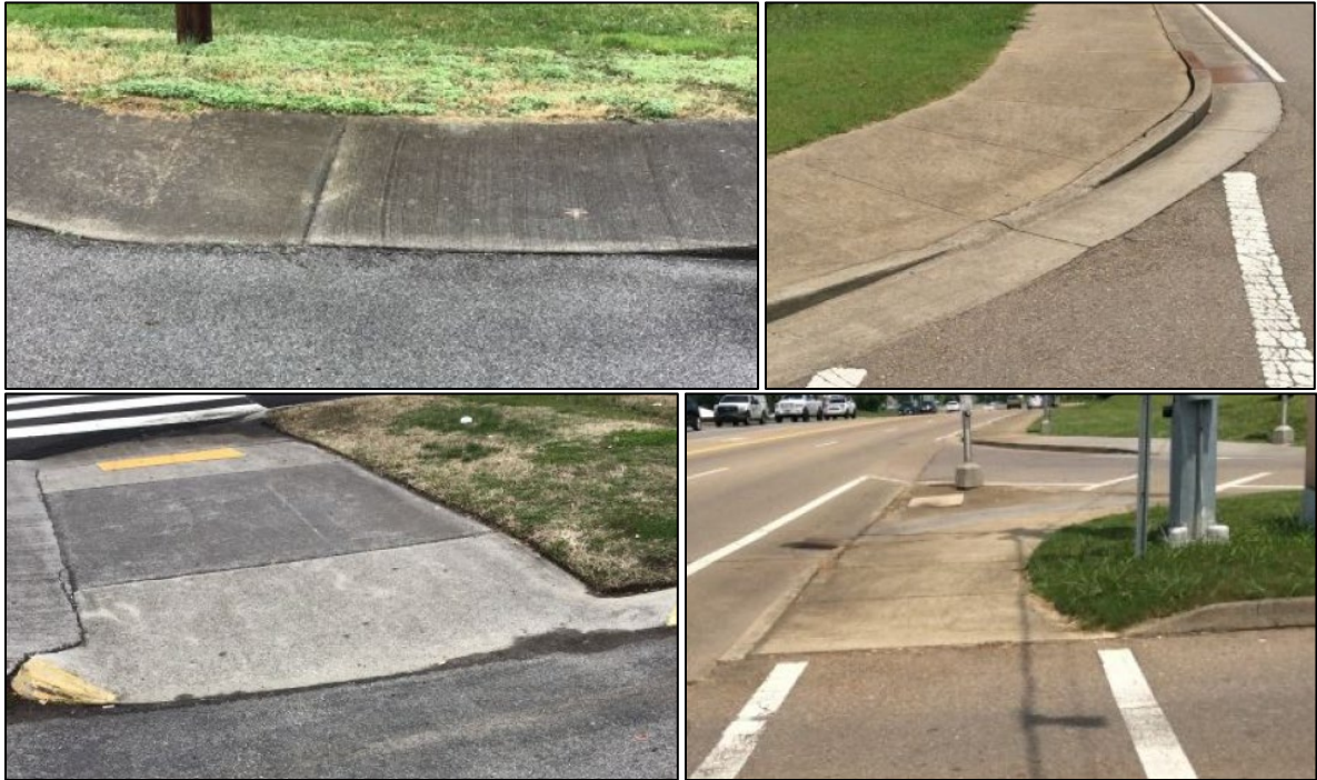
Curb ramps lacking DWs as required or which have low contrast.
