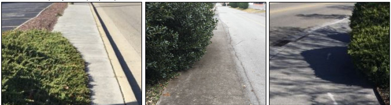
Example of overgrown vegetation that reduces the PAR width to less than 48".
