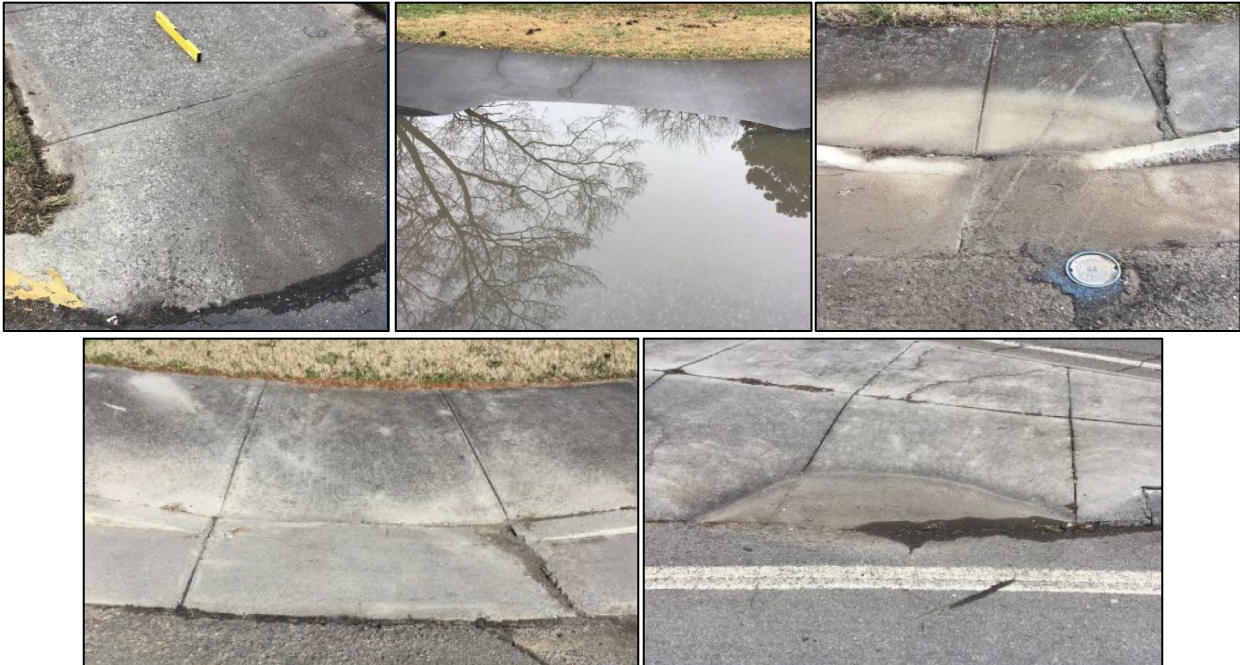
Examples of curb ramps with drainage issues and/or evidence of regular ponding, often with sediment deposition.
