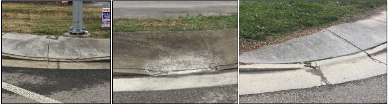
Curb ramps with excessive cross slopes. These ramps also typically have non-compliant landing/TS cross slope.
