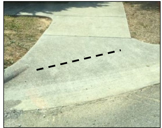
Example of curb ramp that does not provide the required perpendicular grade break.
