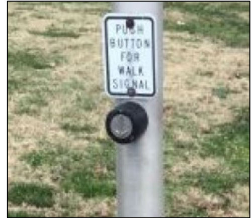
Pushbutton with signage that does not include a crossing direction arrow.
