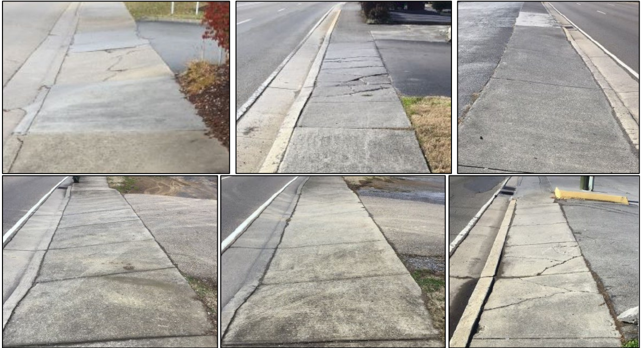
Examples of driveway transitions at the PAR that introduce severe cross slopes and/or vertical elevation changes.
