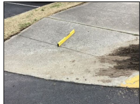
Curb ramp with excessive running slope.
