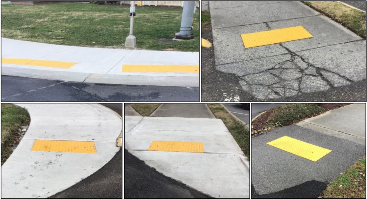
Example of curb ramps with detectable warnings that are not full width of the ramp.
