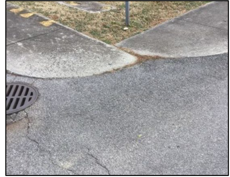
Example of curb ramp with utility structure on the clear space.
