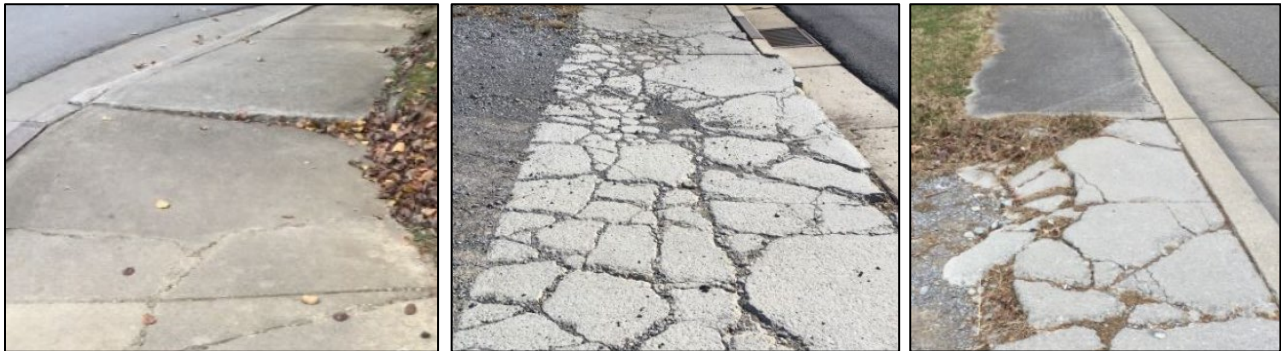
Examples of displacements, separations, and pavement in poor condition in need of maintenance.
