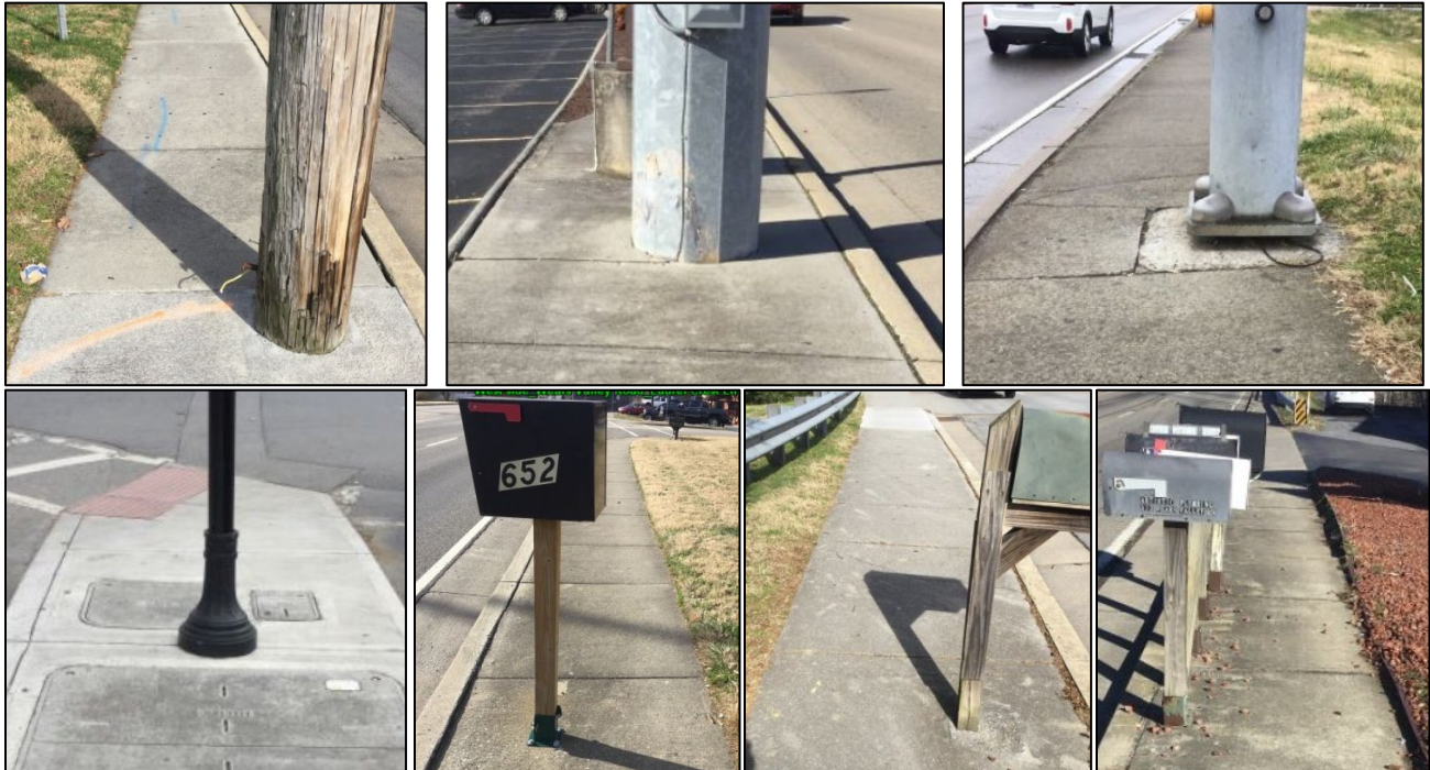
Examples of obstructions of the PAR that reduces the width to less than 48".
