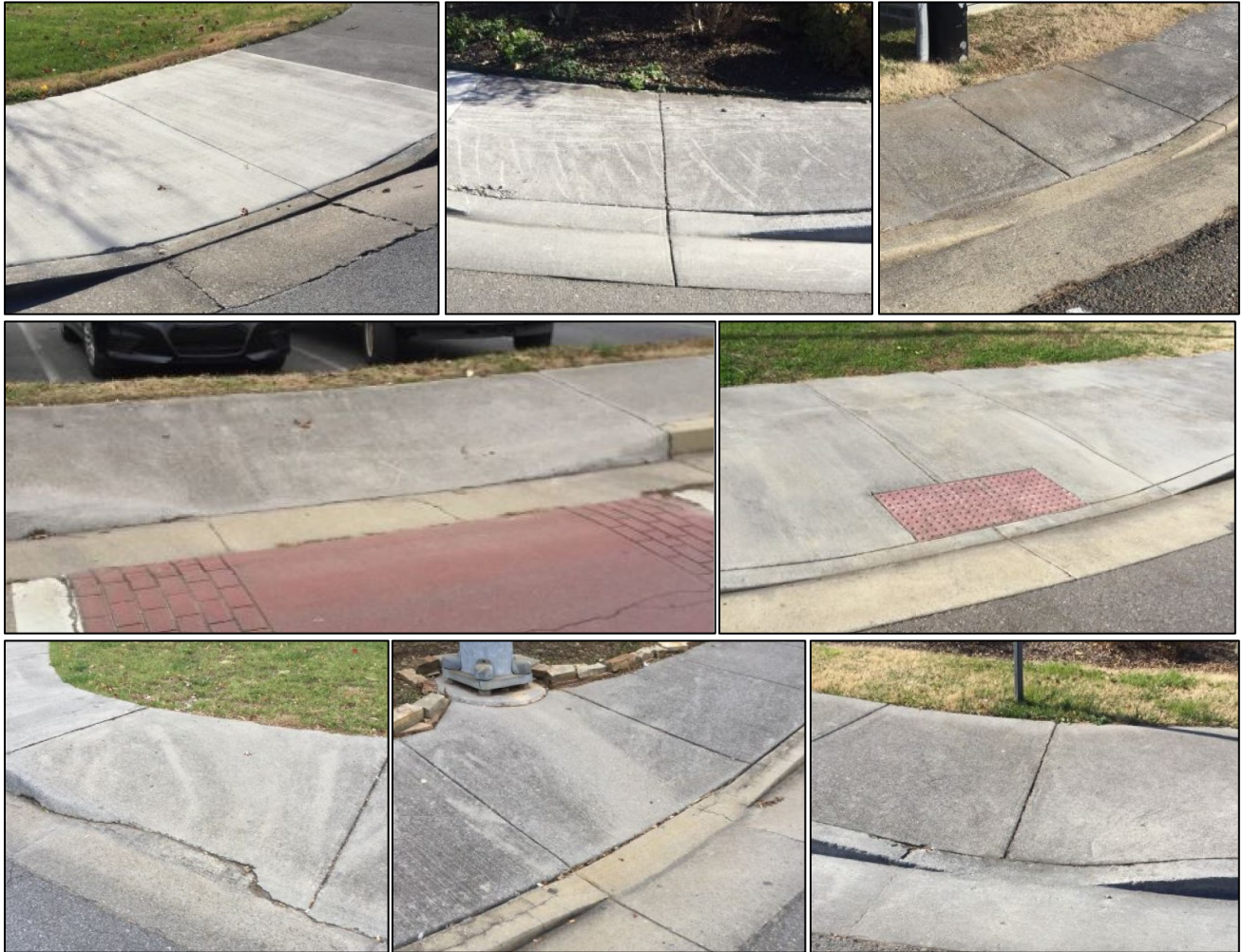
Example of curb ramps that lack a compliant turning space.
