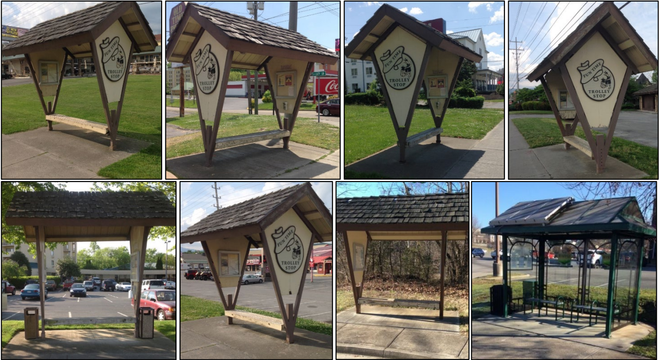
Examples of shelters, with benches that are full width and provide no wheelchair clear space entirely under the shelter.
