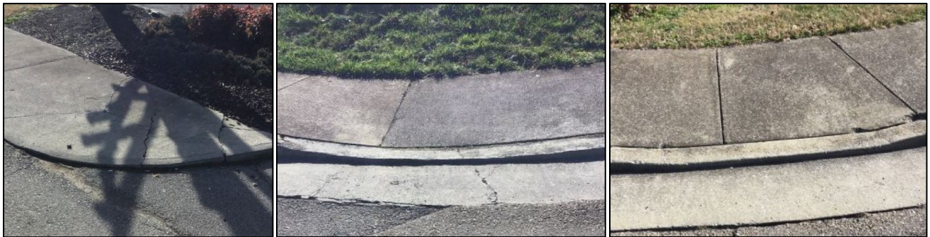
Examples of curb ramps with vertical discontinuities that exceed 1/2" at the curb, on the ramp, or the TS.
