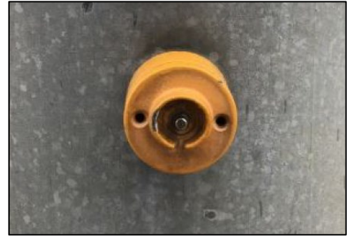
Example of non-compliant pushbutton operable parts (met previous standard)
